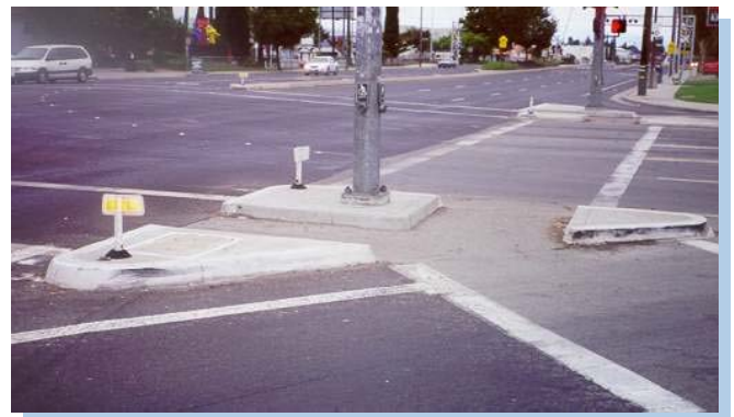
Painted gray concrete pedestrian island
