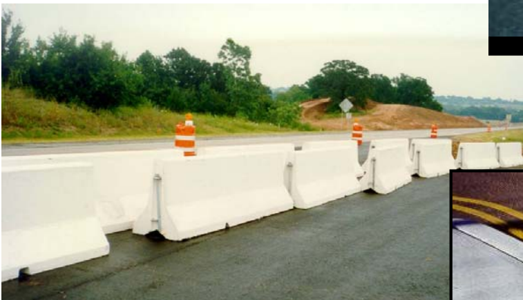
Work Zone Barriers
