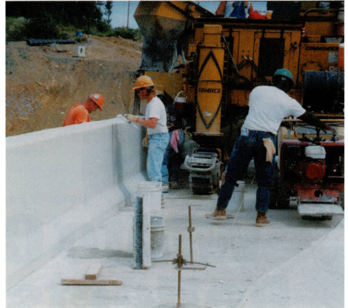
Fig. 2: Finishers follow the slipform paver, filling minor imperfections in a white bridge parapet on the Pennsylvania Turnpike (Photo by Dave Leith, courtesy of Syrstone, Inc.)
