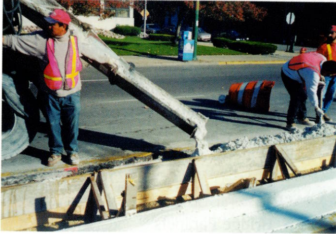
Fig. 3: Workers in Chicago place white concrete curbs for a raised, landscaped median on North Avenue between Larabee and LaSalle Streets (Photo courtesy of Lehigh Portland Cement Co.)
