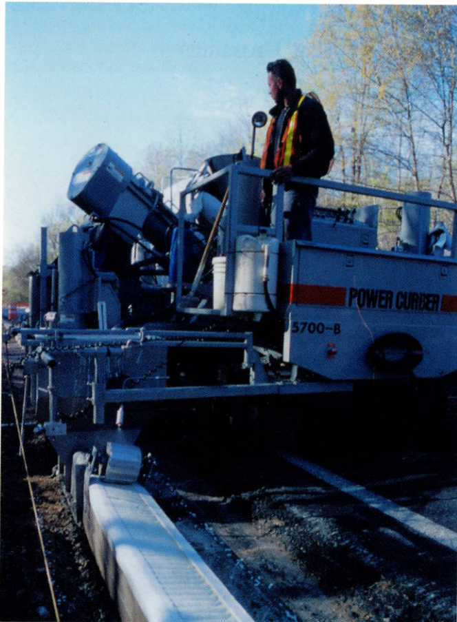
Fig. 4: White grout cap is slipformed on top of the wet gray concrete mountable curb on the Palisades Parkway in New York. An imprinting wheel, attached behind the curber's mold screed, gives the cap facets designed to enhance reflection of the car headlights (Photo © Robert Bailey, courtesy of Power Curbers Inc.)
