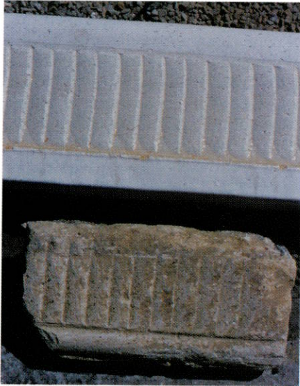
Fig. 5: A section of the faceted new curb (above) and a piece of the weathered old curb below. Palisades Parkway staff members believe the original concrete was white, and they have found it much whiter when they broke open pieces of the old curb
