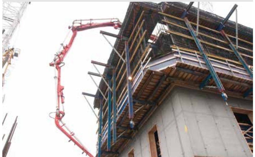
By pressing a button R&S certified staff move the core forms, temporary steps, the placing boom, and a 6-ton crane 16-feet upward to start construction at the next level.
