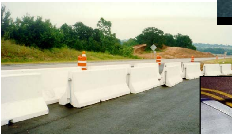
Work Zone Barriers
